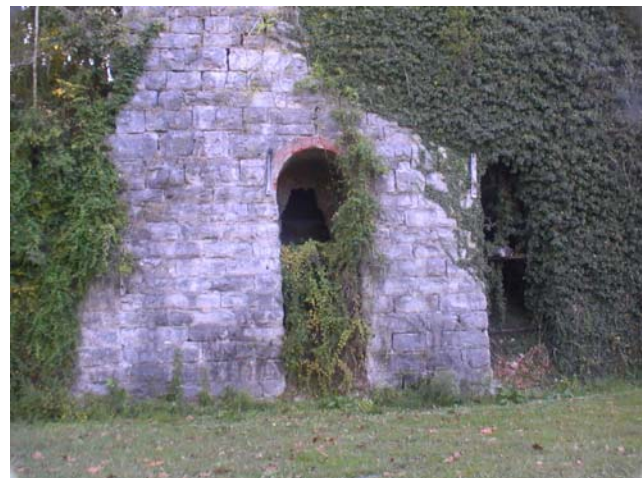
One of the old kilns used to burn limestone and make lime in Milltown. Photo taken on Sept. 19th, 2010 while at the Milltown Community Festival. Spoke there with Ralph Seacat who said Louisville Cement Co. bought the property about 1884 and they built two limestone kilns in 1887 and later added two more which were lined with steel. These kilns are of historical value to Milltown and Crawford County.
