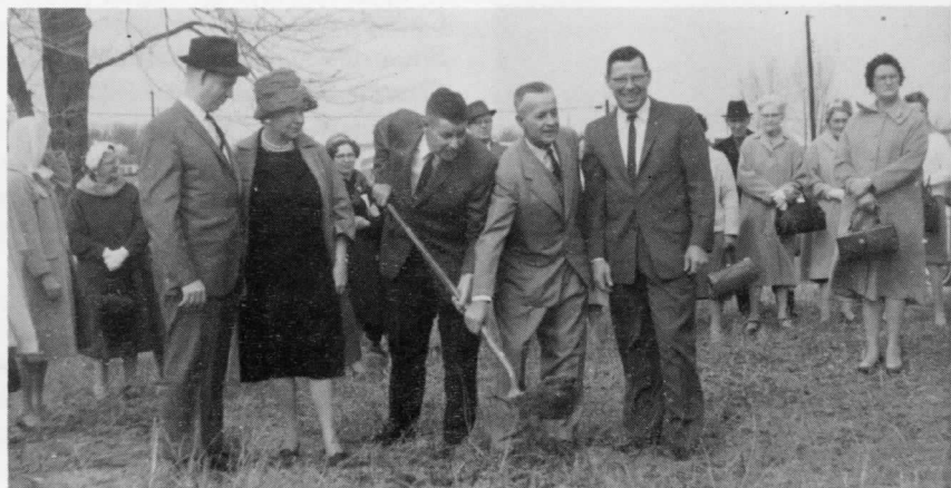
The 1963 ground-breaking ceremony for the new church parsonage on Maddox Street for Rev. Earl and Faye Vaughn.
