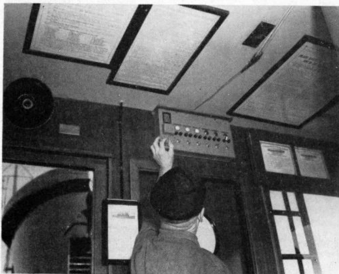
Skipper Hasbrouck checks tow and position light control panel on wheel house wall. Note radio loudspeaker
