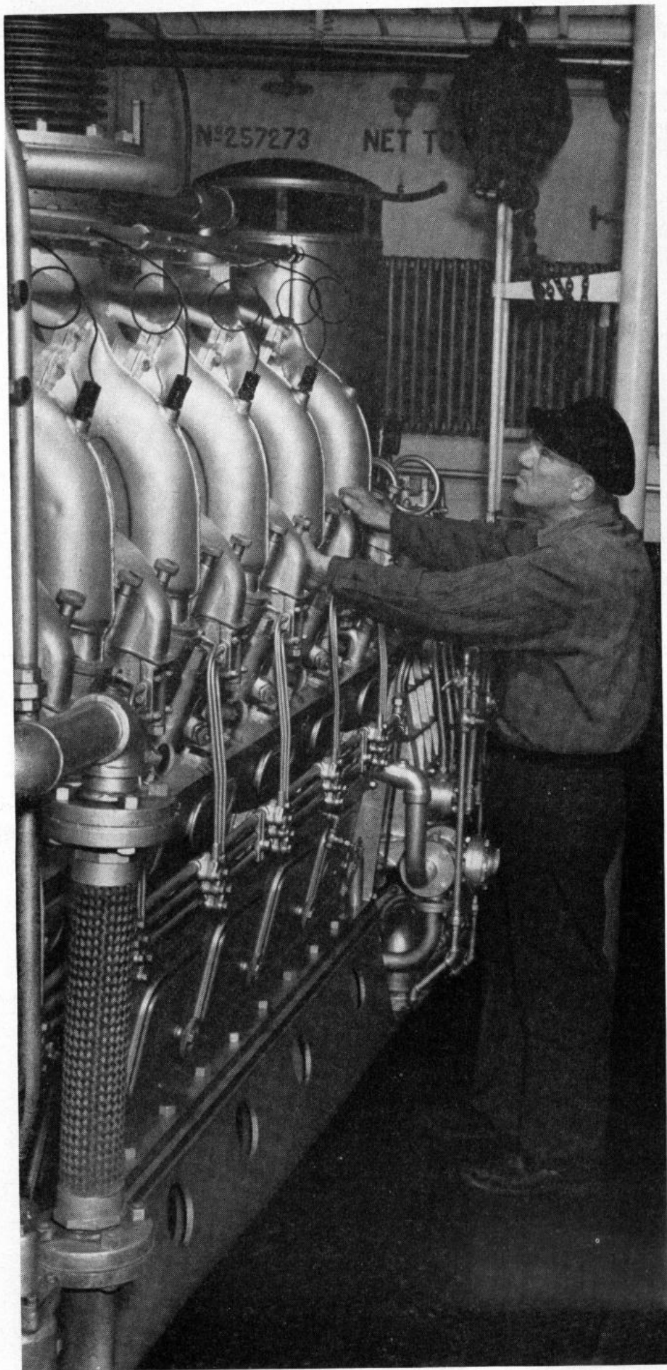
Engineer "Patty" Goode critically takes the pulse of 1200-horses-worth of dazzling diesel in the Paterson's power room
