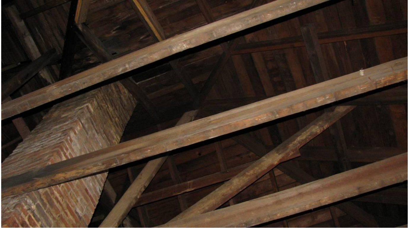
Renovation of the depot has exposed the rafters supporting the roof over the waiting rooms. On the left is the waiting rooms' chimney.
